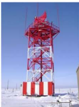
Primary Surveillance Radar Antenna
